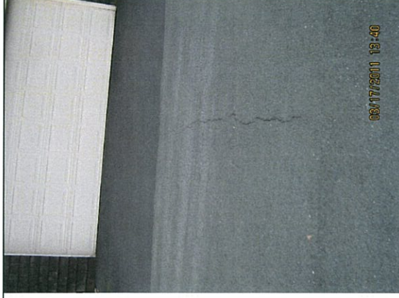
Photo 6: Photo taken March 17, 2011 showing crack that starts in the driveway reflecting through the overlay, as it did pre-construction.
