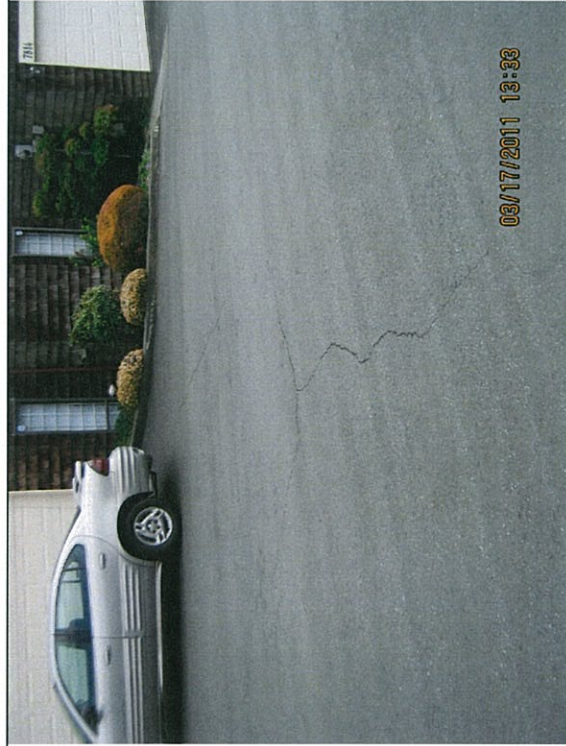
Photo 5: Photo taken March 17, 2011 showing crack reflecting through the overlay from the original crack as seen in Photo 2.
