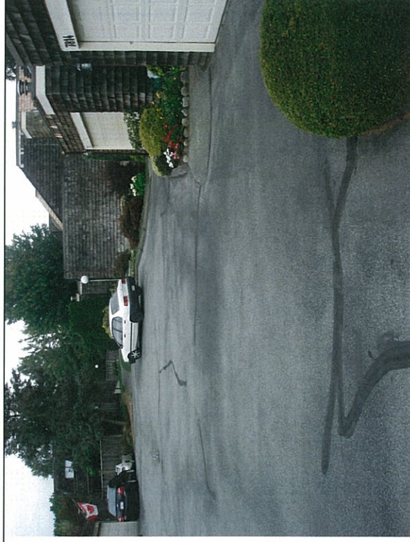
Photo 2: Photo dated March 4, 2009 of the north end of Marchwood cul-de-sac, showing pre-existing asphalt cracks present.
